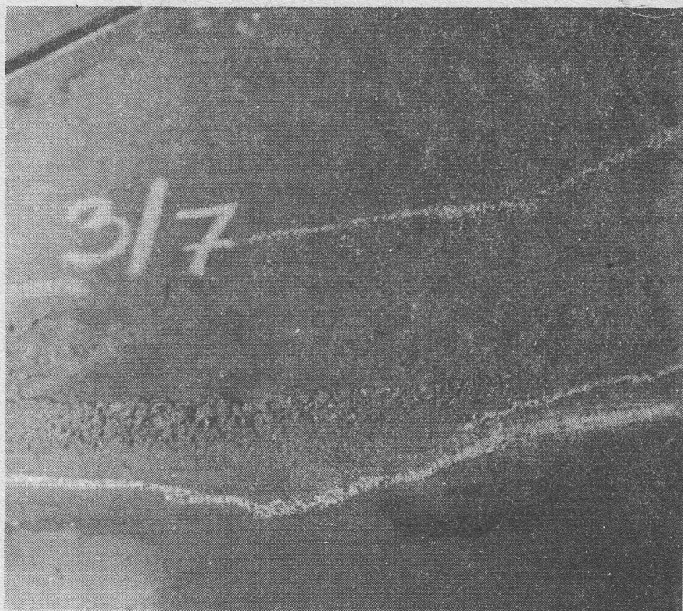
Fig. 1f. Damage of runner hub padded with stainless steel (reversible machine, pumped-storage power plant at Żarnowiec)
